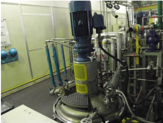
Picture 4: Production equipment at Plant 2. Fire is strictly prohibited because of the presence of flammable liquids.
