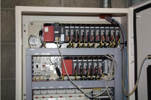
Pictures 6 and 7: The ZCT (Pic 6) mounted on the cables at the base of the panel board sends leakage current information to the insulation monitoring module “QE82LG” (Pic 7) within the panel board for processing.
